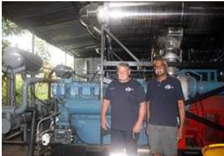
Above: Inkulu Plastic Piping MD Gabriel Reddy and factory manager Paul du Preez take a breather after commissioning the generators,
